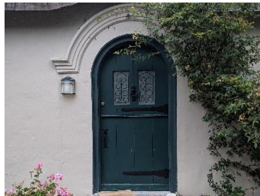
Front door to be restored.
