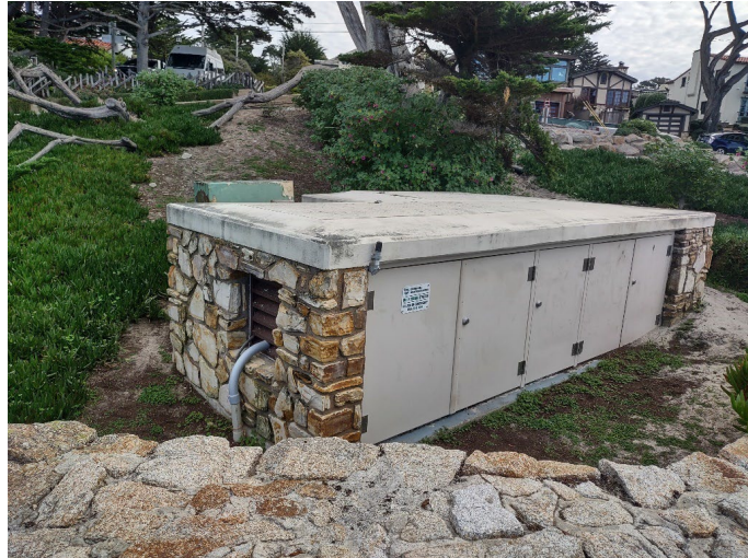
Wastewater lift station near 8 th Avenue
