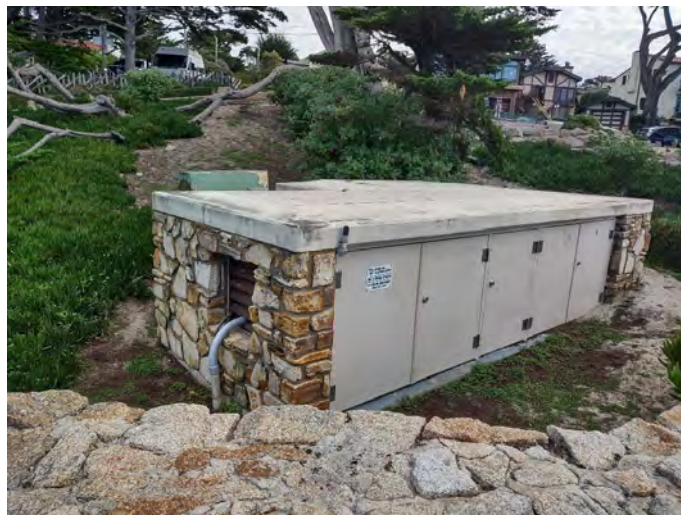
Wastewater lift station near 8 th Avenue
