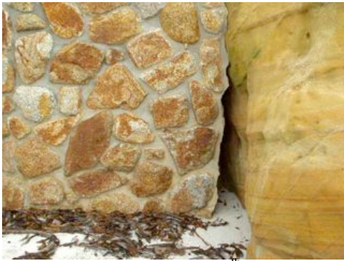
Gap in seawall between 13 th & Santa Lucia (2004)
