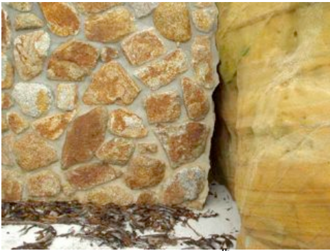
Gap in seawall between 13 th & Santa Lucia (2004)
