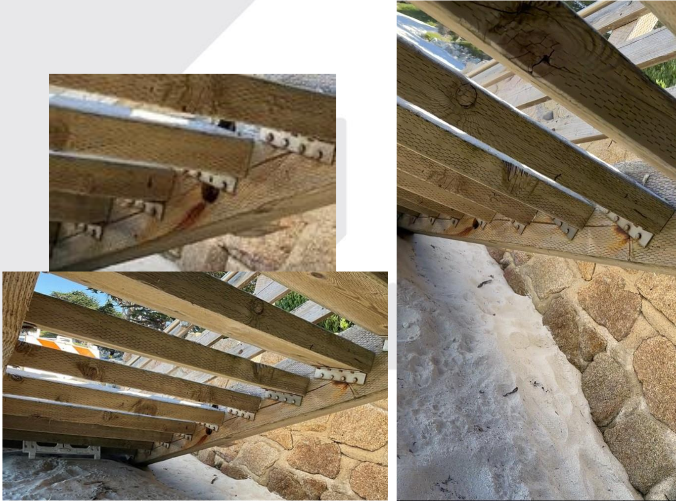
Figure 9: Stair 7 Split Stringer at Countersunk Post Connections Replace (2) 6x12 Stringers
