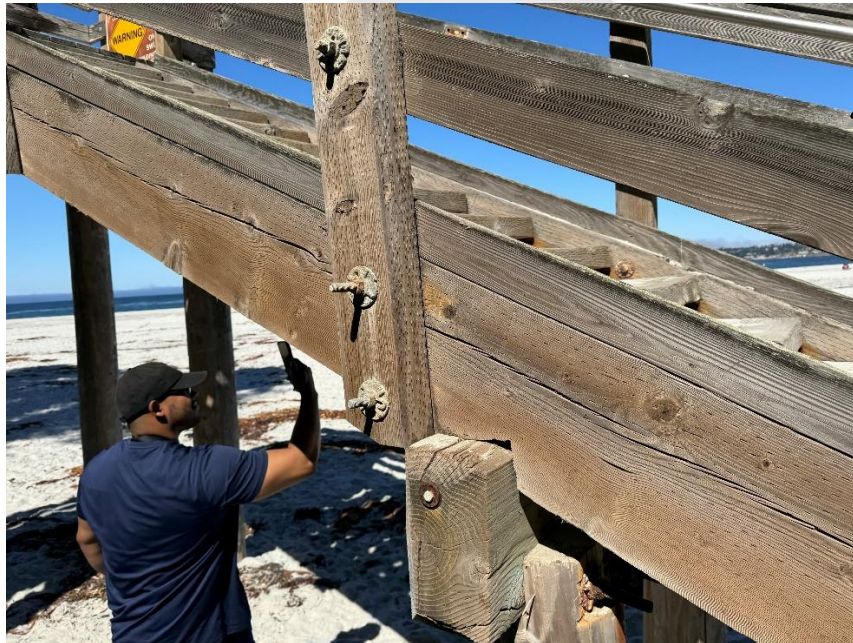
Figure 6: Stairway 4 Split Stringer from Middle Landing to Beach
