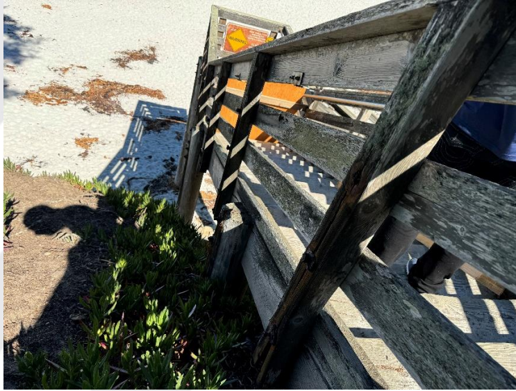
Figure 3: Stair #4: Guardrail Post Upper Flight to Landing
