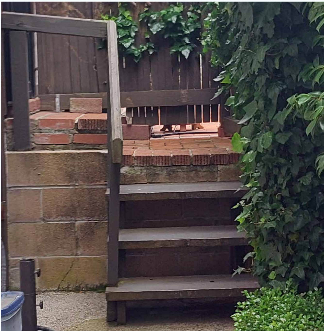
STAIRS AND RAIL TO BE REPAIRED
