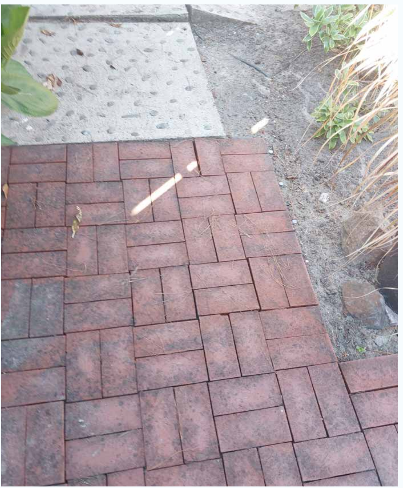
BRICK PAVING TO BE REPAIRED
