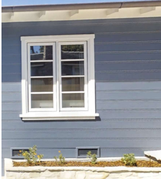
EXISTING HOUSE IMG NOTE: ALL EXTERIOR SIDING REPAIR AND COLOR TO MATCH EXISTING
