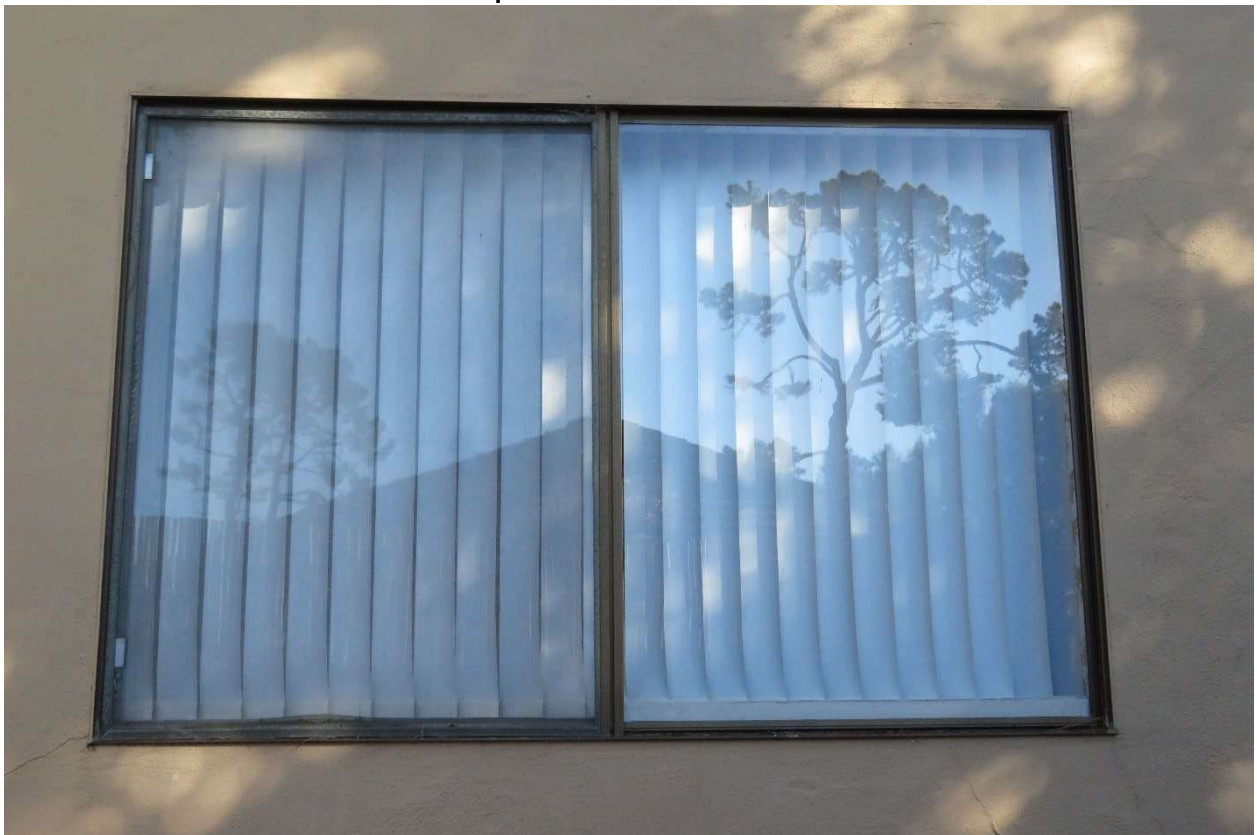
Window #5 - master bedroom - to be replaced
