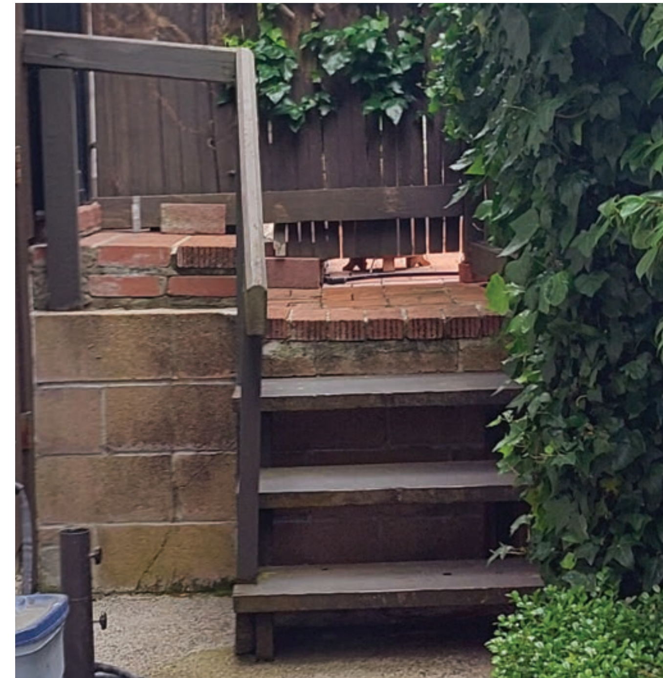
STAIRS AND RAIL TO BE REPAIRED
