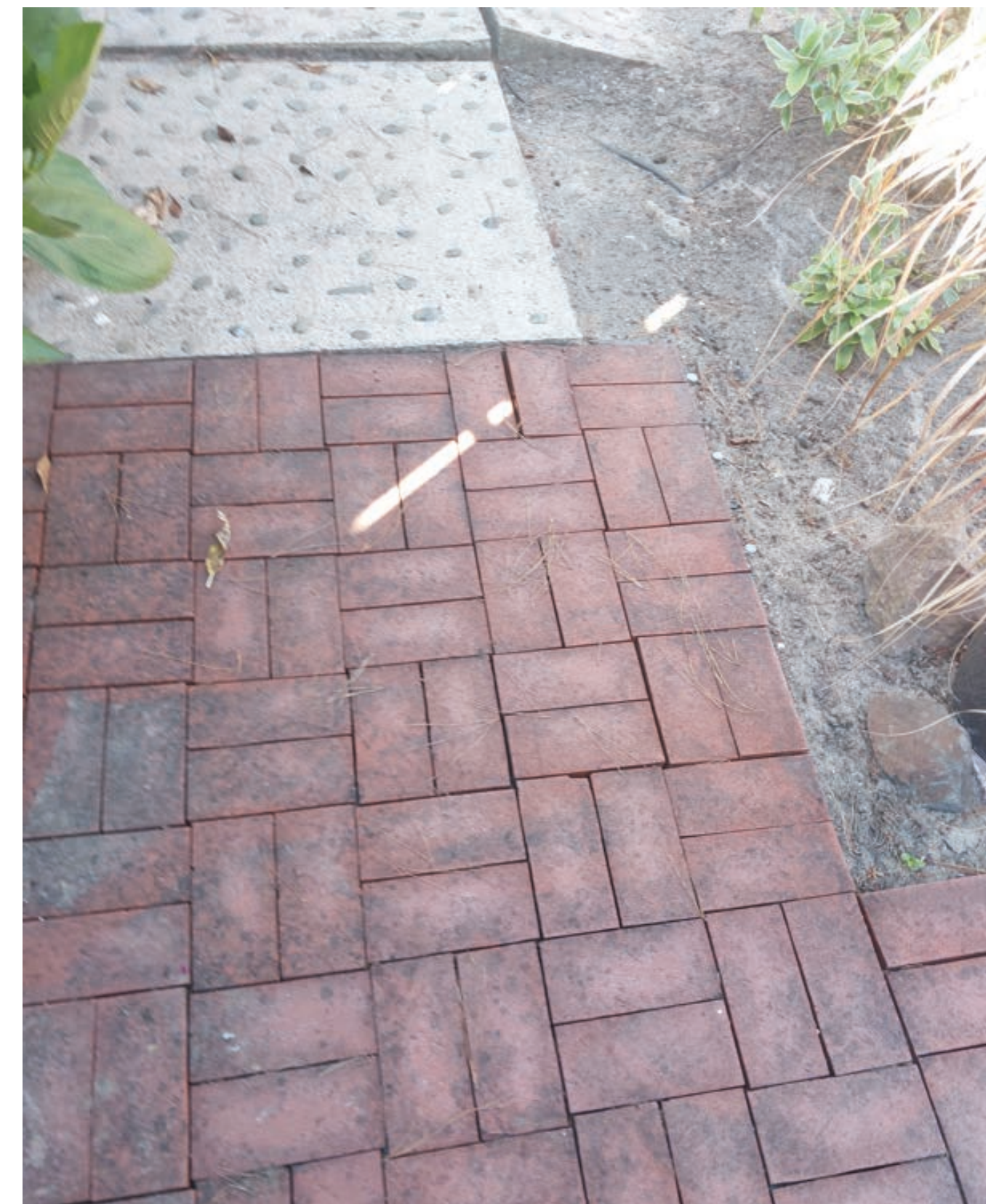
BRICK PAVING TO BE REPAIRED
