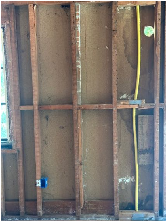
Failed waterproofing, BR fixture
