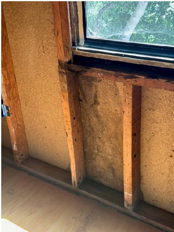
Failed waterproofing, BR windows
