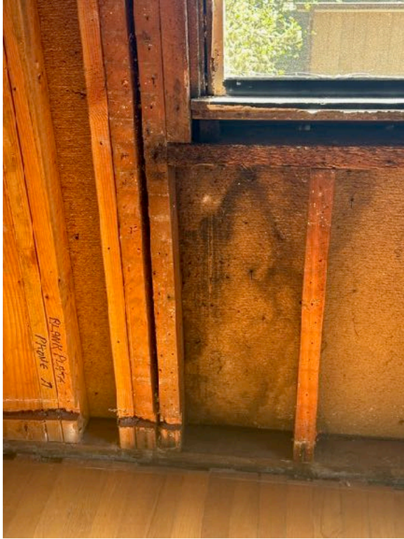
Failed waterproofing, BR windows
