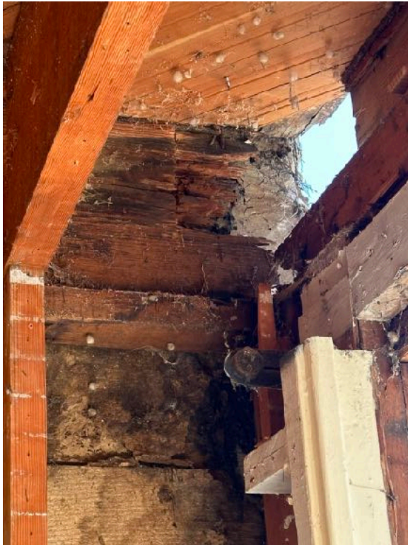
Interior view of dry rot damage
