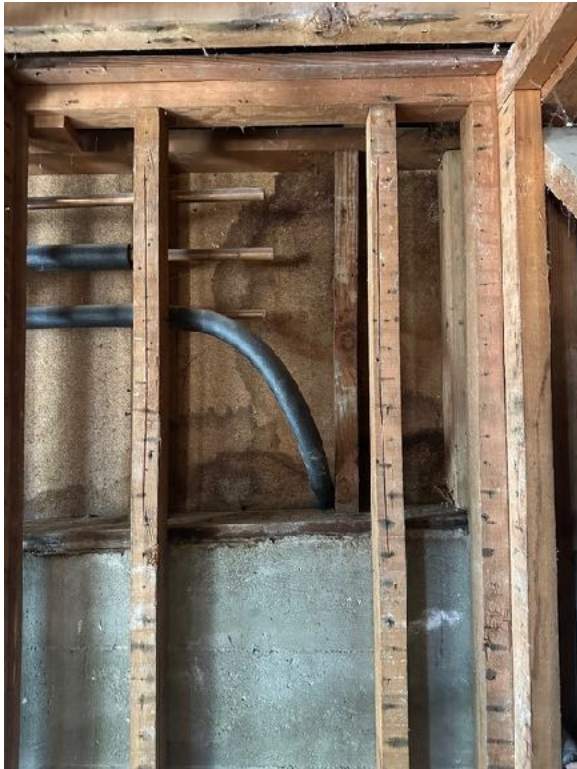
Failed waterproofing, first floor north
