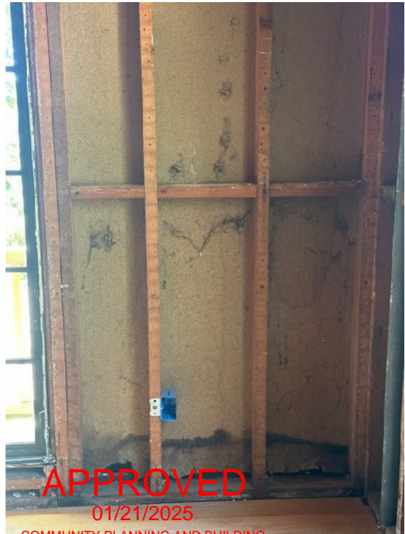
Failed waterproofing, BR door
