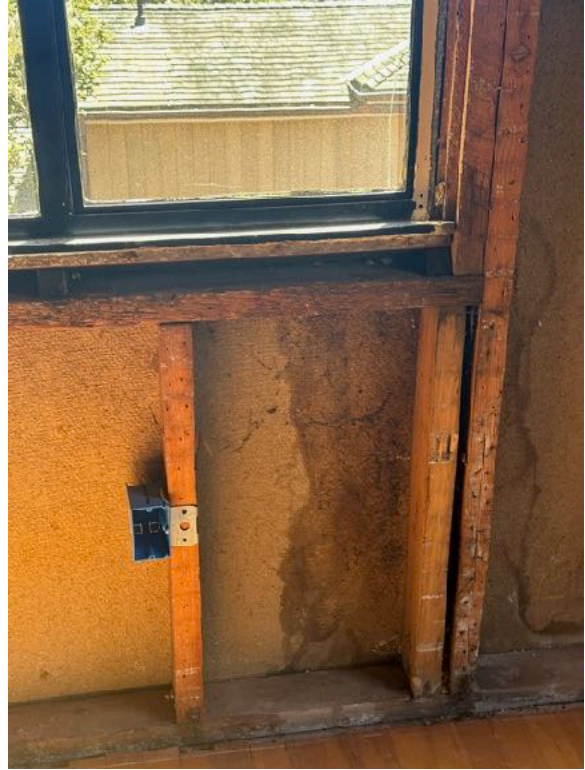
Failed waterproofing, BR windows
