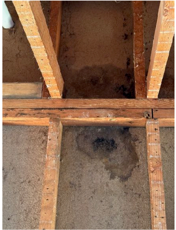
Failed waterproofing, attic south
