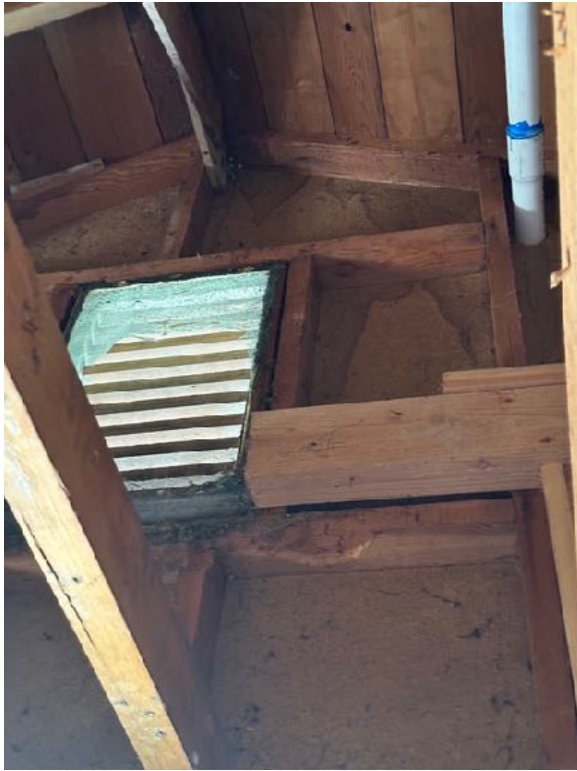
Failed waterproofing, attic south
