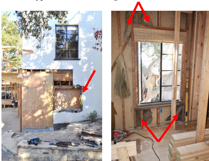
Figures 1 and 2. Left image shows the south elevation at the southwest building corner, showing extensive rot and stucco deterioration. Right image shows typical moisture infiltration patterns around the windows.
