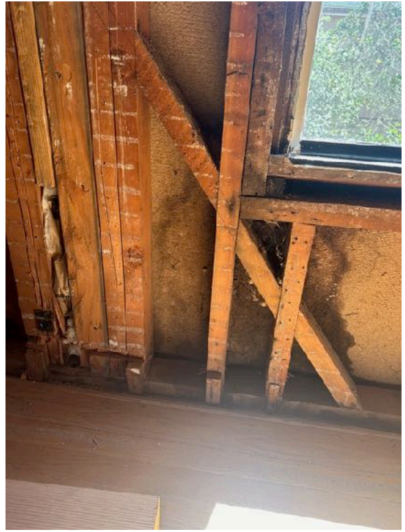
Failed waterproofing, LR windows
