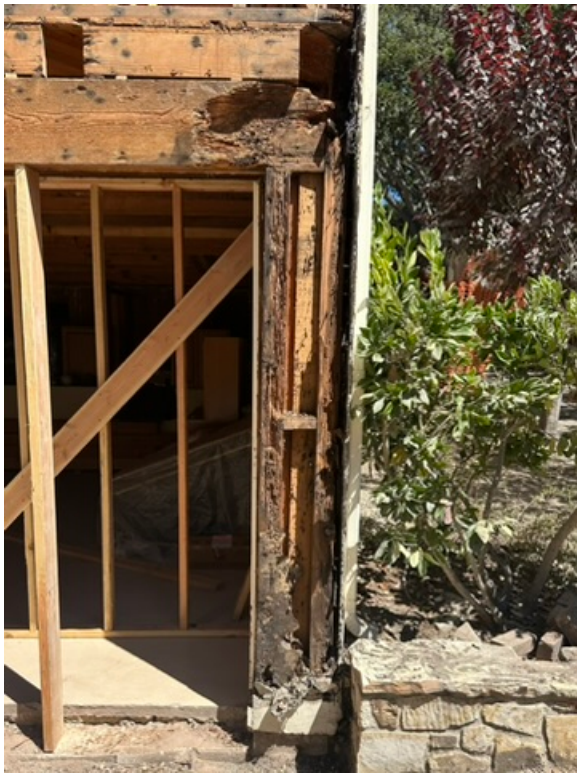
West facing garage door post
