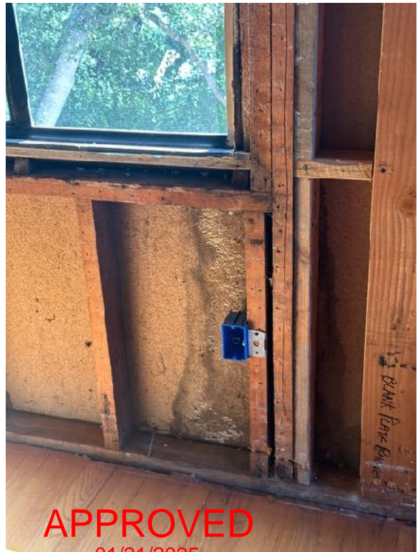
Failed waterproofing BR windows
