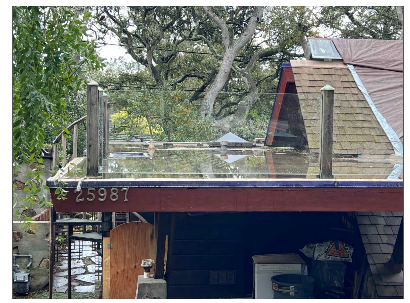
FLAT ROOF DRAINAGE ISSUE PHOTO NTS
