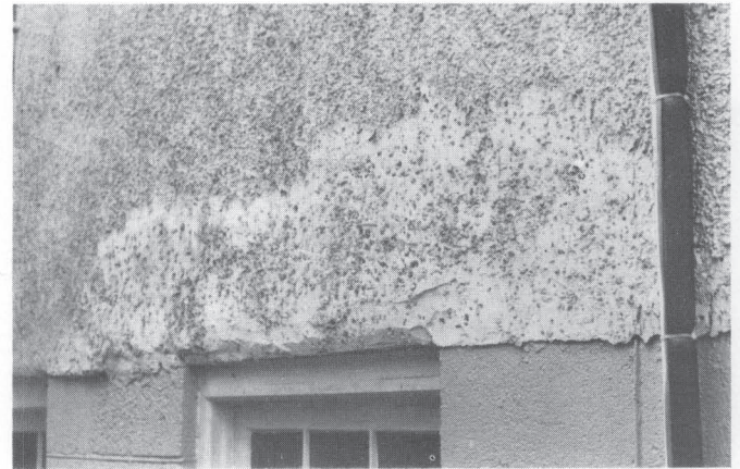
Fig. 14. This poorly executed patch is not the work of a professional plasterer. While it may serve to keep out water, it does not match the original surface, and is not an appropriate repair for historic stucco. Photo: Betsy Chittenden.
