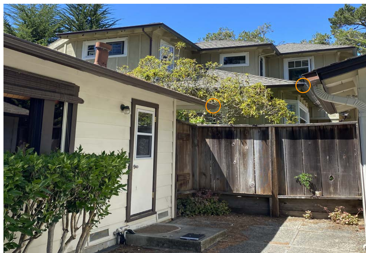
VIEW FROM PATIO SHOWING EAVE HEIGHT DIFFERENCE W/ NEIGHBOR
