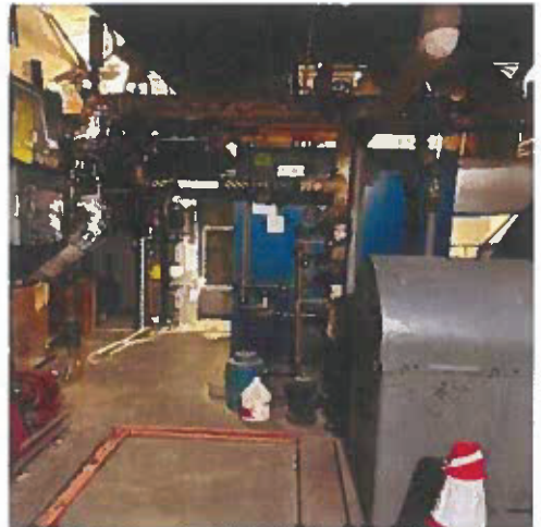
Figure 17 - Existing Hot Water Boiler (Mechanical Room)
