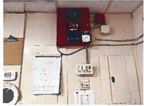
Figure 39 - Existing Fire Alarm Control Panel
