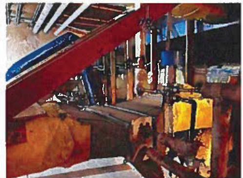
Figure 29 – Existing Hot Water Heating Coil Temperature Control Valve (TCV) in Attic
