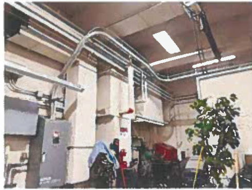
Figure 23 – Existing Hot Water Pipes Over Transfer Switch
