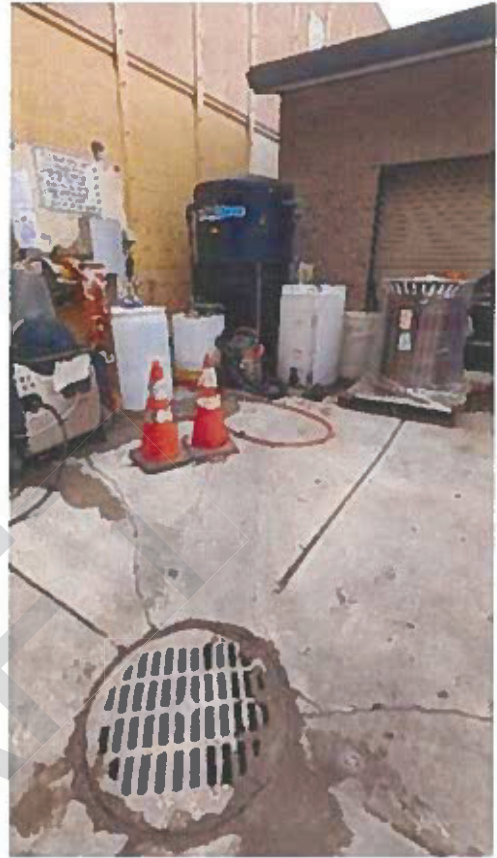
Figure 16 - Existing onsite storm drain recycled water system
