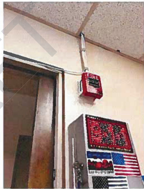
Figure 40 - Existing Manual Pull Station
