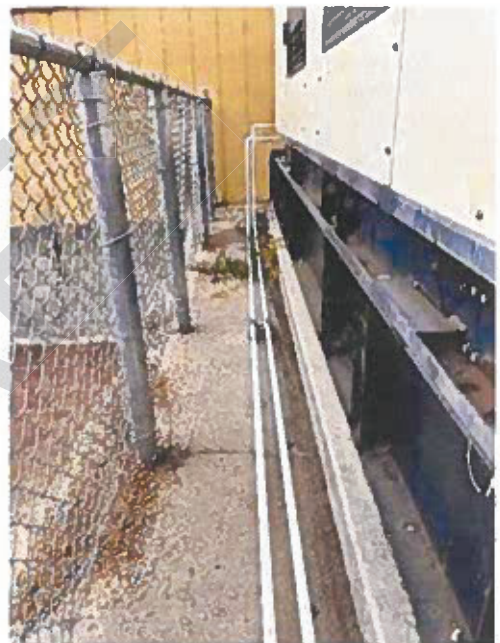
Figure 37 - Clearance in front of existing generator
