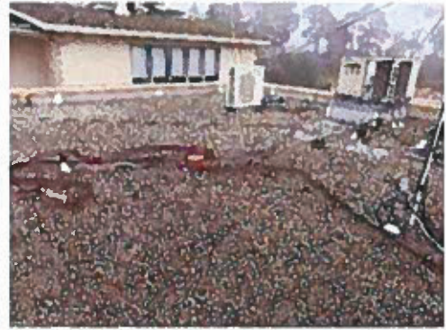
Figure 33 – Existing disconnected lightning protection
