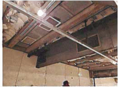
Figure 26 – Existing Shooting Range Exhaust Ventilation
