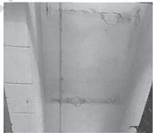
Figure 14 – Moisture stains through cracks in existing concrete slab
