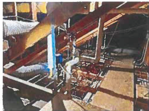
Figure 32 – Electrical splices not in electrical box.
