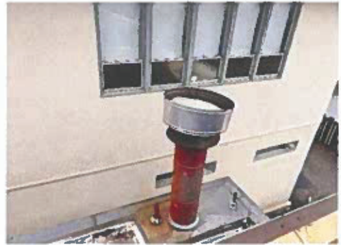
Figure 22 – Existing Hot Water Boiler Flue
