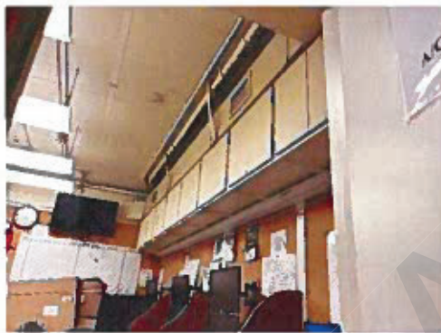
Figure 28 – Existing Shooting Range Supply Ventilation
