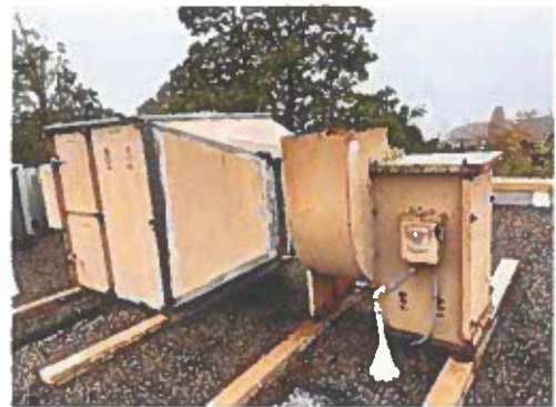
Figure 25 – Existing Shooting Range Exhaust Fan/Filtration Unit
