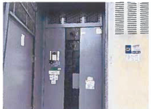
Figure 38 - Existing power distribution switchboard
