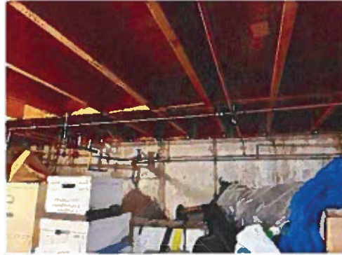
Figure 19 – Garage Storage - Existing Uninsulated Hydronic Piping
