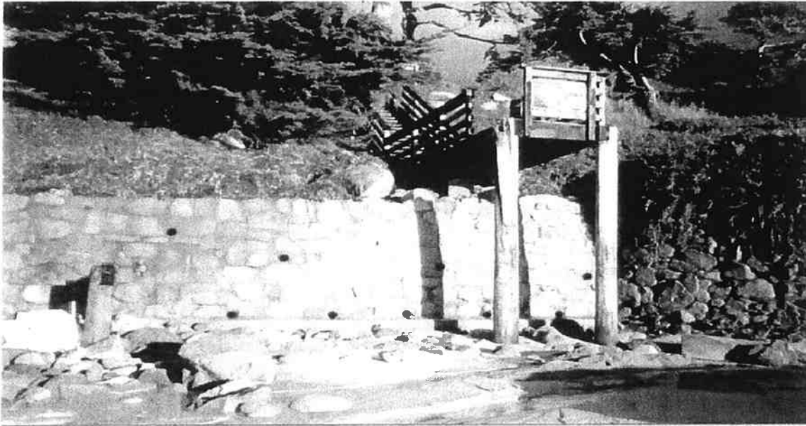
Photo 6 – Limited Damage to the Upper Portion of the Break-Away Stairs at Tenth Avenue (North)
