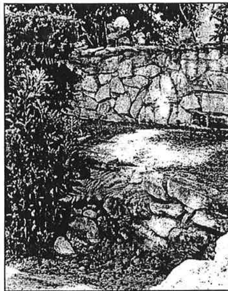
Each individual wall should not exceed four feet in height. Terrace or step walls on steeper slopes and locate plantings in front of each terrace when feasible.
