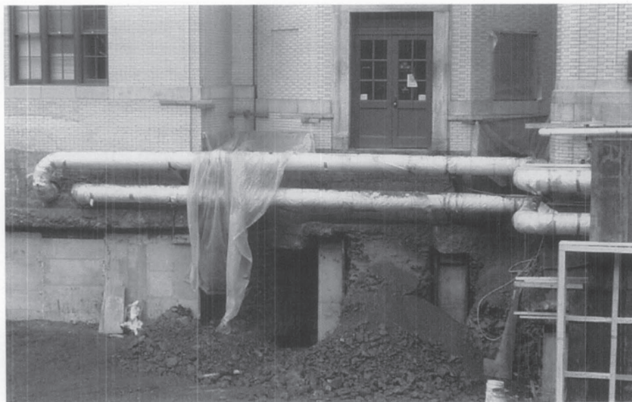
Figure 3. Concrete pier underpinning to an existing building may be necessary when adjacent construction occurs. In this example, pits are hand dug beneath the foundation of the historic building to provide space for wood forms. After concrete is poured into the forms, the space between the top of the pier and the bottom of the original foundation is packed with a quicksetting grout. The historic building owner should retain an independent engineer to ensure that the underpinning plan adequately protects the historic structure. Photo: Professor Arpad Horvath, Department of Civil and Environmental Engineering, University of California, Berkeley.
