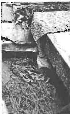
Clogged gutter leading to corrosion.
