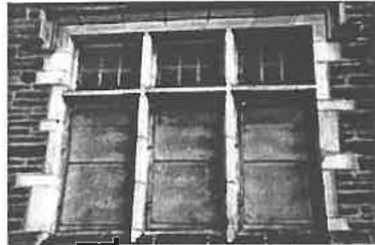
Deteriorated lower window sash shown prior to its replacement in kind.
