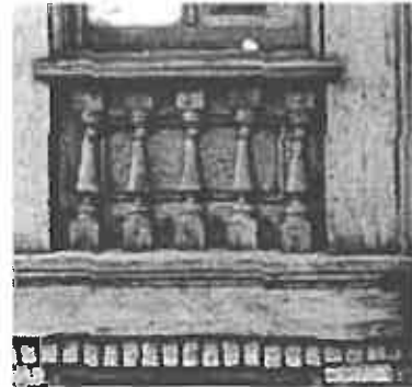
Wood features inappropriately stripped of traditional painted finish.
