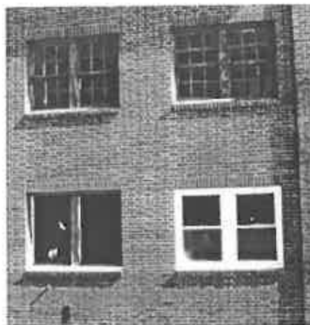
Incompatible new window (lower right), resulting in loss of the building's historic character.
