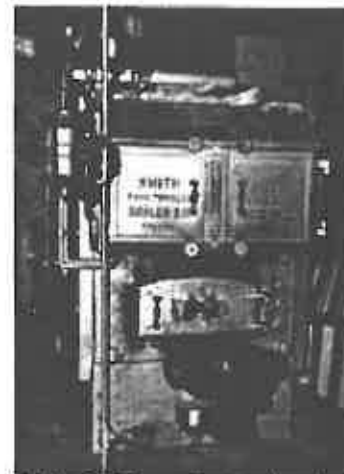
Boiler kept in good operational condition through ongoing maintenance.
