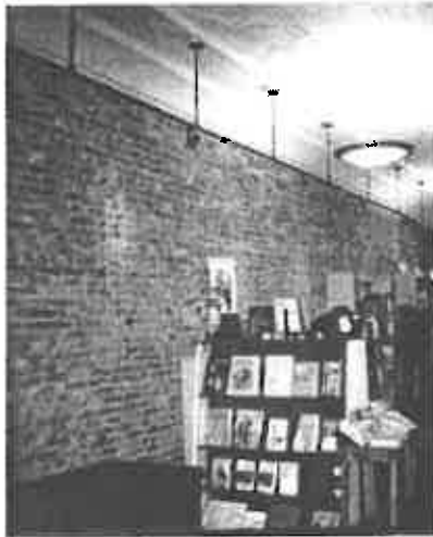
Exposed brick wall after inappropriate removal of historic plaster.
