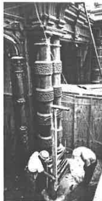
Missing cast-iron elements replaced with cast aluminum.
