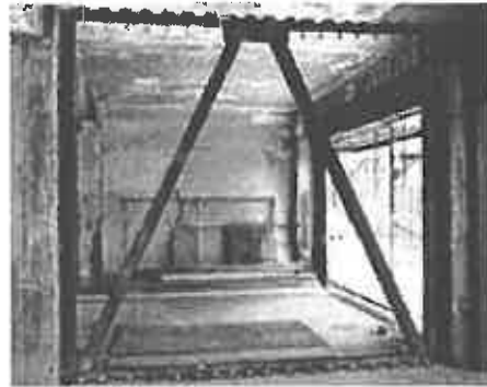
Structural brace installed between piers as seismic reinforcement to be concealed within re-built wall.
