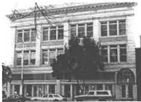
Replacement awning design incompatible with the building's historic character.
