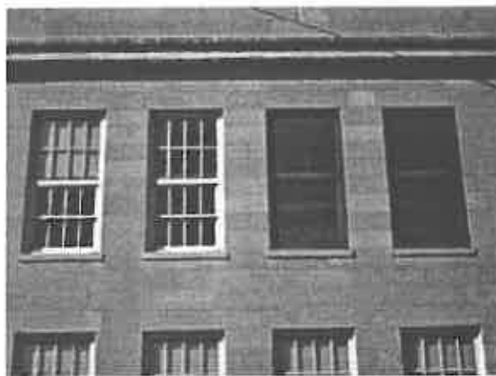
Historic windows (left) on primary elevation inappropriately replaced with tinted glazing (right). Photo: Mike Jackson.
