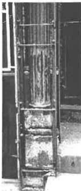
Cast iron column revealed during removal of non-significant storefront.
