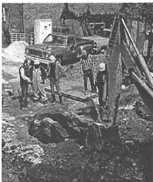
Inappropriate excavation causing damage to historic building foundation.
