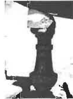
Surviving baluster of terrace that provides a prototype to replace damaged balusters.
