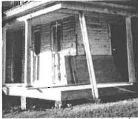
Deteriorated porch resulting from inadequate maintenance requires repair.
