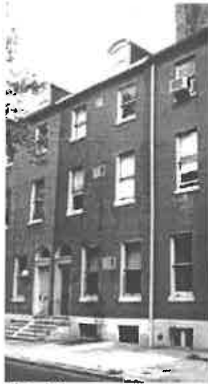
Historic building material destroyed by through-the-wall air-conditioners.
