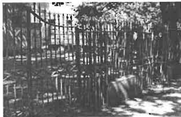
Historic Iron fence to undergo repairs and refinishing as part of rehabilitation work.
