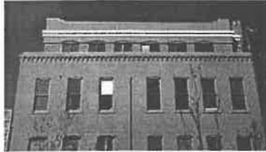
Rooftop addition that dramatically changes the appearance of the historic building.
