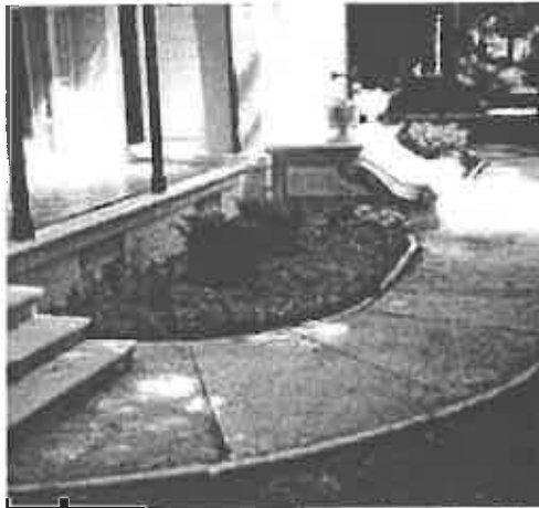
Deteriorated limestone walkway to be replaced in kind.
