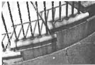
Chemical reaction between new concrete steps and historic iron railing that causes unsightly appearance.
