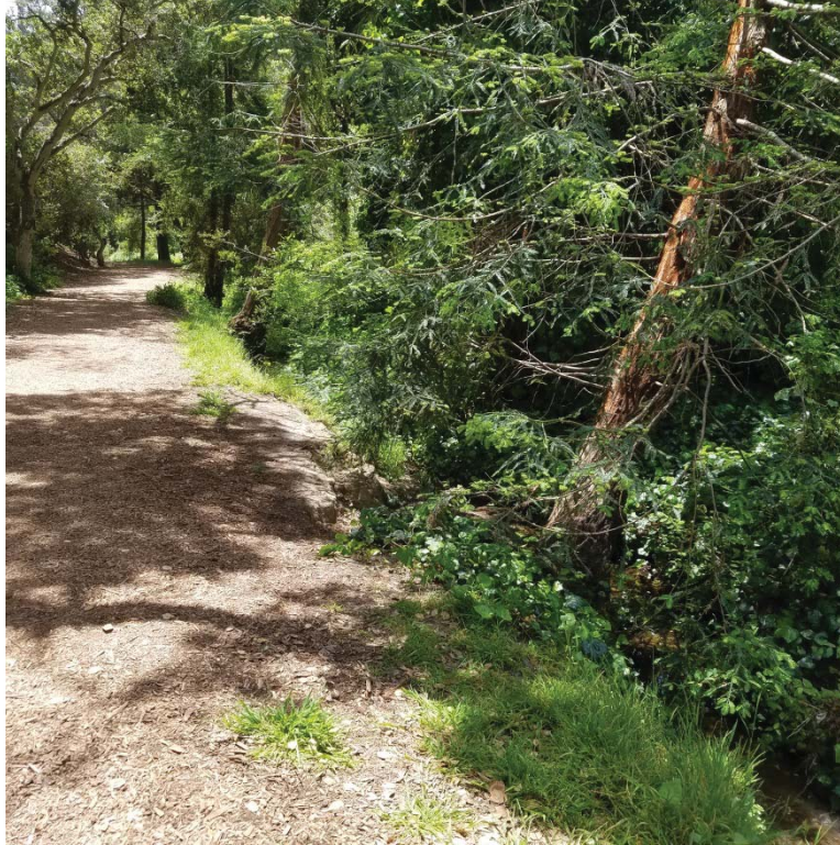
Photo 3: Looking in southerly direction along Serra Trail. Note creek immediately adjacent to the road and trees beginning to fail into creek as a result of channel incision and bank erosion.
