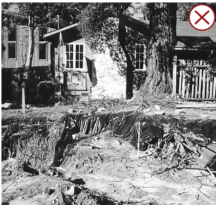
Excavation work shall be planned to avoid significant impacts to root systems. As shown here, cutting into major roots systems without City approval will weaken or even kill a tree and is unlawful.
