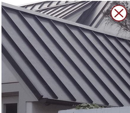
Standing seam metal (inappropriate)
