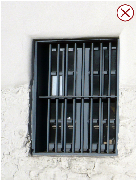
Security bars that are permanently mounted on the exterior are inappropriate.
