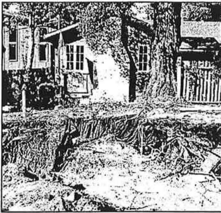
Excavation work should be planned to avoid significant impacts to root systems. As shown here, cutting into major roots systems without City approval will weaken or even kill a tree and is unlawful.
